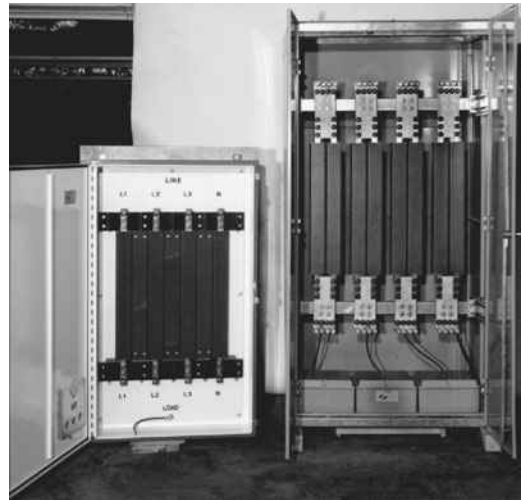
Figure 14.18 Interior view of a high-capacity hybrid power conditioner. (Courtesy of Control Concepts.)
